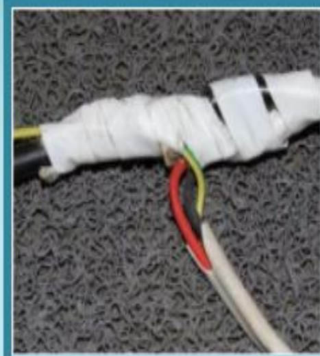
Exposed Electrical Parts
